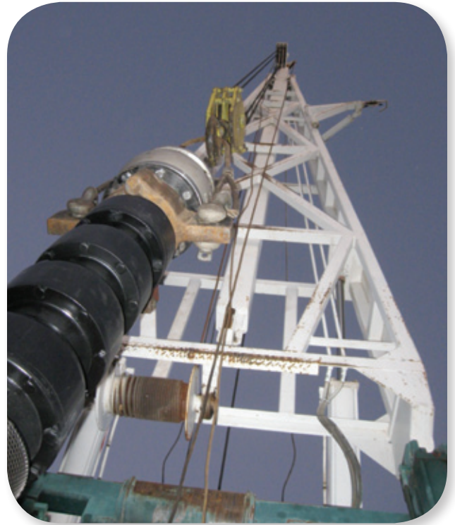
Photo of the installation of a new deep well submersible pump at the San Ricardo Well.
